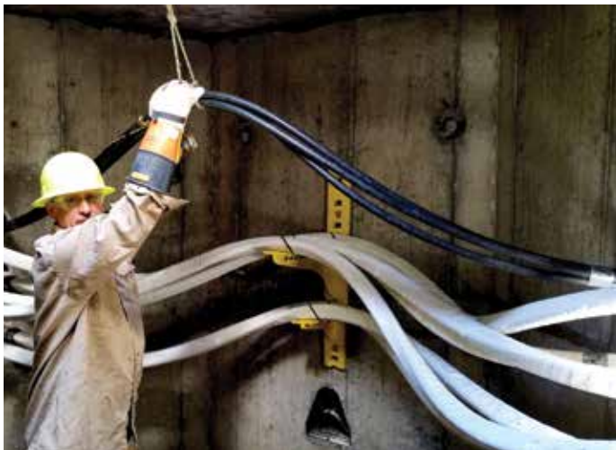
A portion of the loop feed system.
