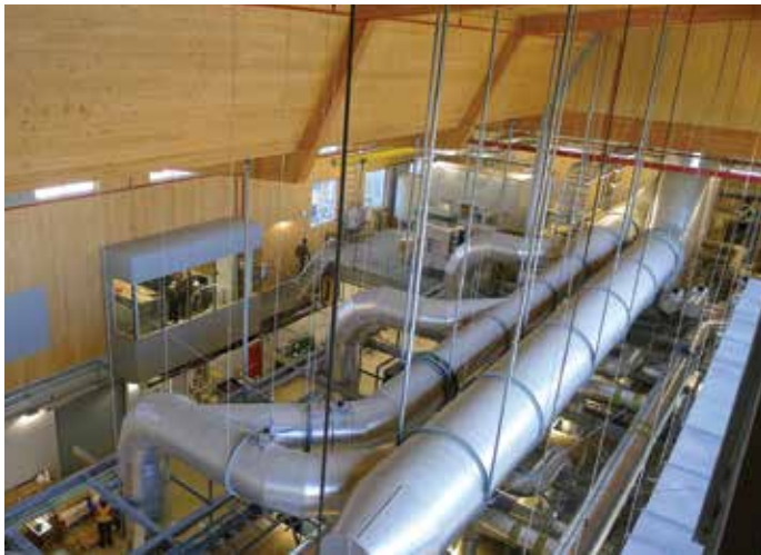
UBC's new Campus Energy Center.
