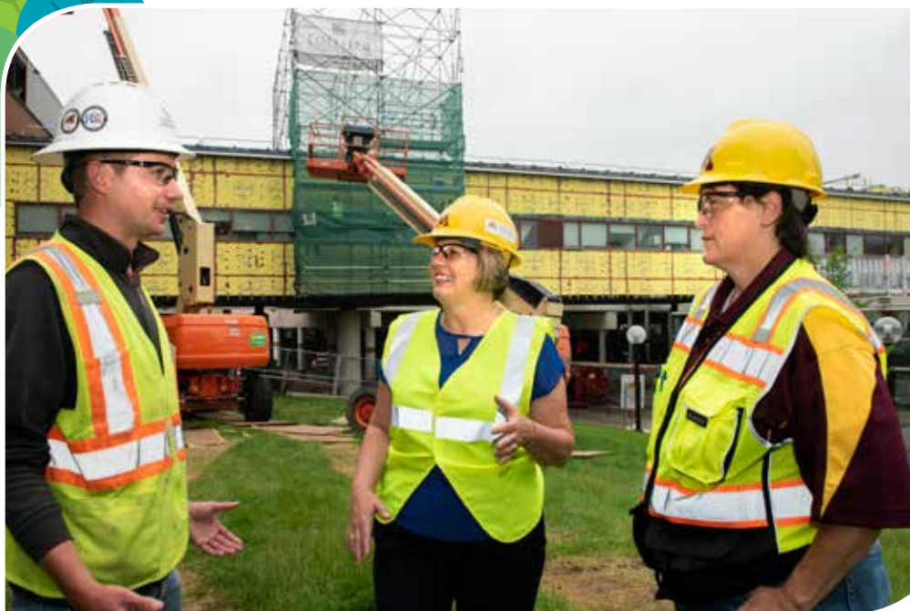
Manlet, center, discusses West Bank Student Union Skyway exterior resurfacing project with Sawyer Stecher of Loeffler Construction, left, and Karen Haakonson, right, U of M project manager.
