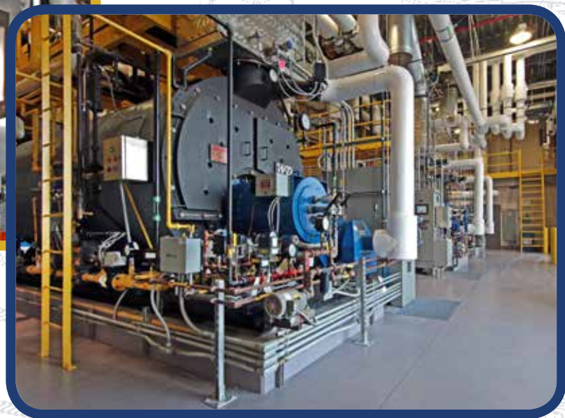
Photos courtesy of Preferred Utilities Manufacturing
