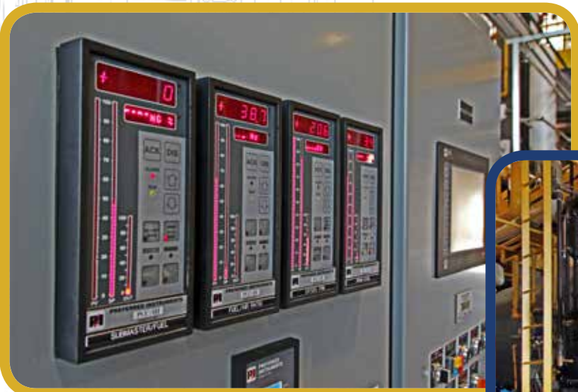
Monitoring panels and new boiler at the VA Medical Center in Erie, Pennsylvania.
