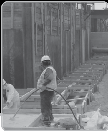
THERMAL ENERGY CORP (TECO) CHP EXPANSION PROJECT GILSULATE®500XR HAS BEEN THE SYSTEM INSULATING/PROTECTING TECO'S STEAM/COND./PUMP COND. FOR 25 YEARS! "FAILURE IS NOT AN OPTION FOR TECO."
