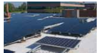
Photovoltaic Roofing System on White Reflective Roof
