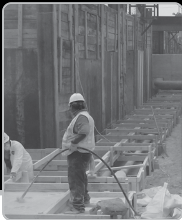
THERMAL ENERGY CORP (TECO) CHP EXPANSION PROJECT GILSULATE®500XR HAS BEEN THE SYSTEM INSULATING/PROTECTING TECO'S STEAM/COND./PUMP COND. FOR 25 YEARS! "FAILURE IS NOT AN OPTION FOR TECO."
