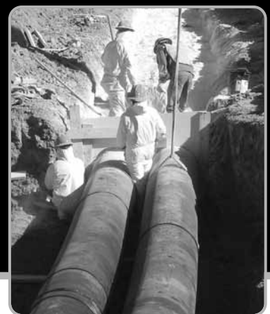
NATIONAL CENTER THERAPEUTICS MANUFACTURING - TEXAS A&M 24" HDPE CWSR INSULATED WITH GILSULATE ® 500XR. A&M'S CAMPUS DISTRIBUTION MASTER PLAN FOR CWSR/HWSR RECENTLY CHANGED FROM PIP TO GILSULATE ® 500XR
