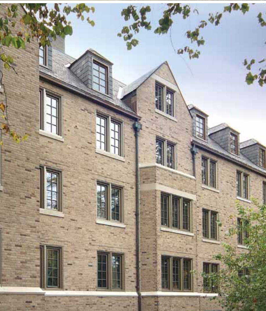
University of Notre Dame's historic Farley Hall renovation. The existing window frames were left in place and encapsulated with aluminum interior trim to preserve and restore the campus' architectural legacy.
