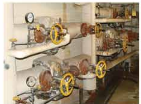
Bare Pipe Fittings
