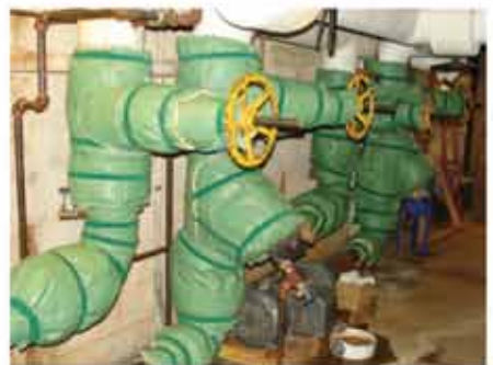
Pipe Fitting Components Insulated with Cut 'n Wrap
