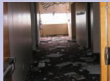
Miller Center hallway. This was typical interior damage.
