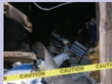
Maintenance Tech building WITH aircraft that caused explosion and fire.
