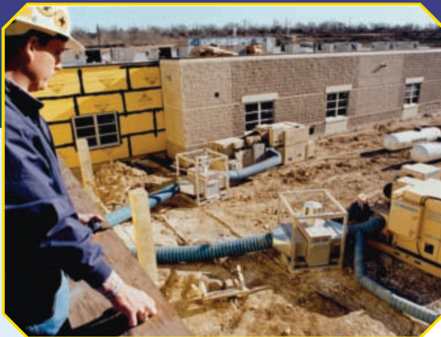
Desiccant dehumidification underway at an elementary school construction site near Austin, Texas.
