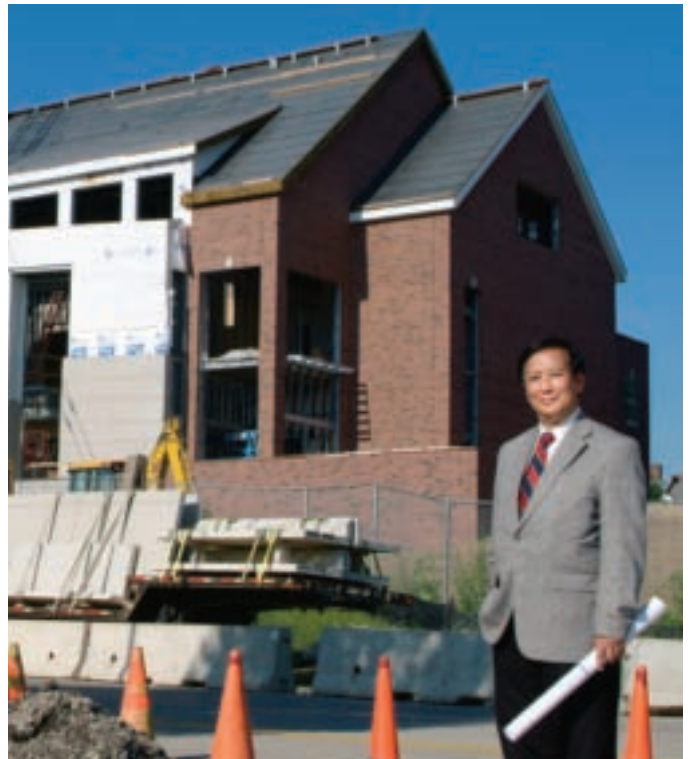
Nearing completion is ISU’s Student Success Center, which will highlight academic and athletic achievements and services.
