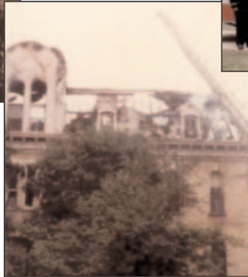
Workers were installing a sprinkler system in St. Edwards Hall when this fire started. Unfortunately, the sprinklers were not functional yet.
